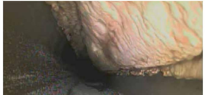
Figure 1. Carbonaceous soil build up in an evaporator tube.
