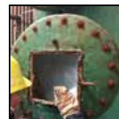
Figure 2: Scrubber depressurized allowing for more treated air volume
